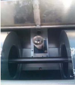
Figure 2 AtmosAir model FC100 inside unit ventilator serving Classroom 120
